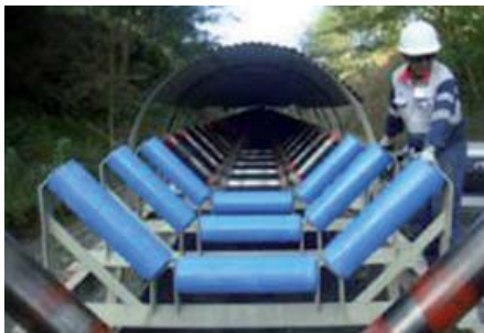
Photo PT Newmont. Installation of the UCC rollers on the 6km conveyor that connects the mine to the treatment plant.
